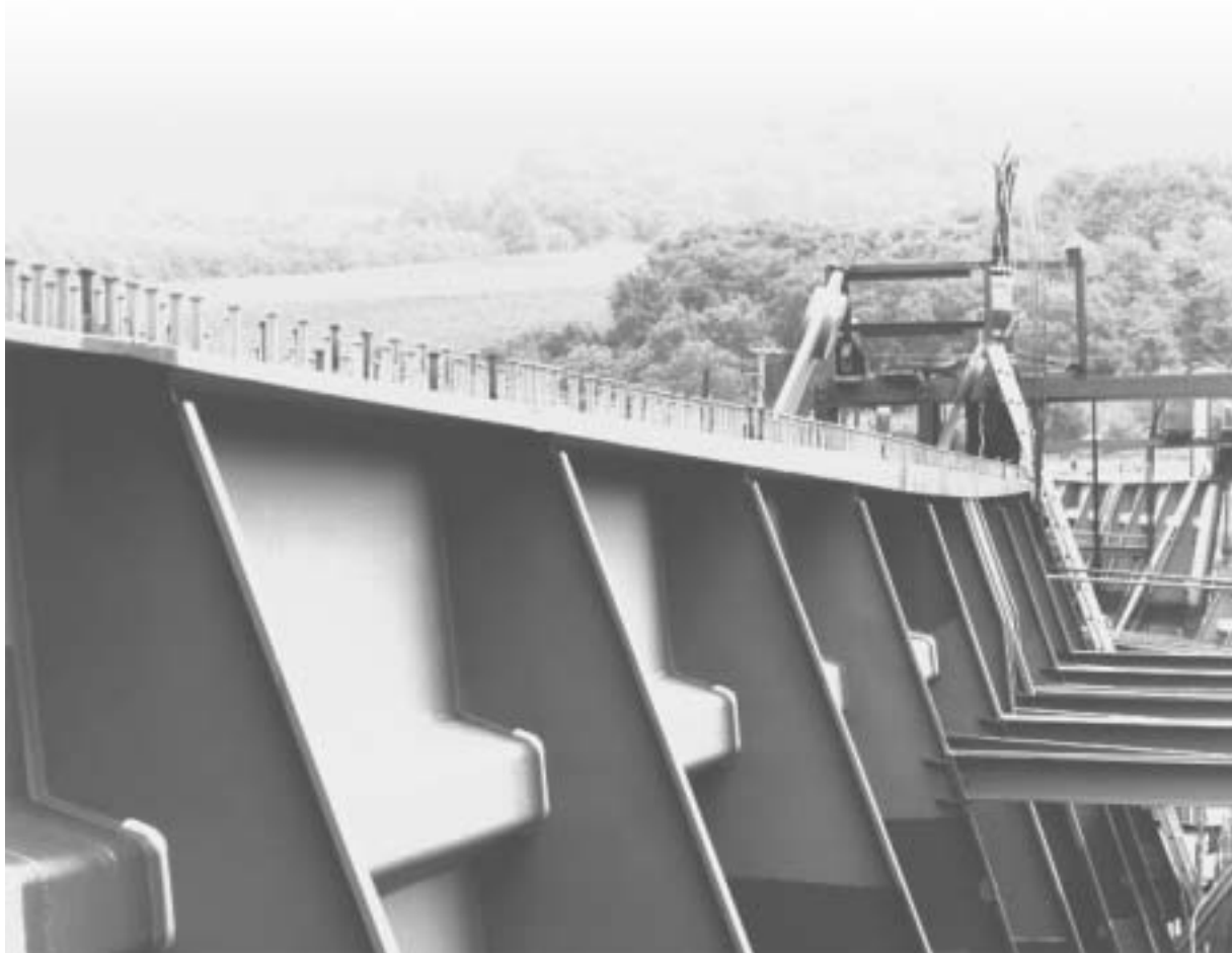
The top chord of the Mosel bridge at Schengen, Luxembourg: 1,100 t of S355N LP-Plates in thicknesses up to 140 mm
