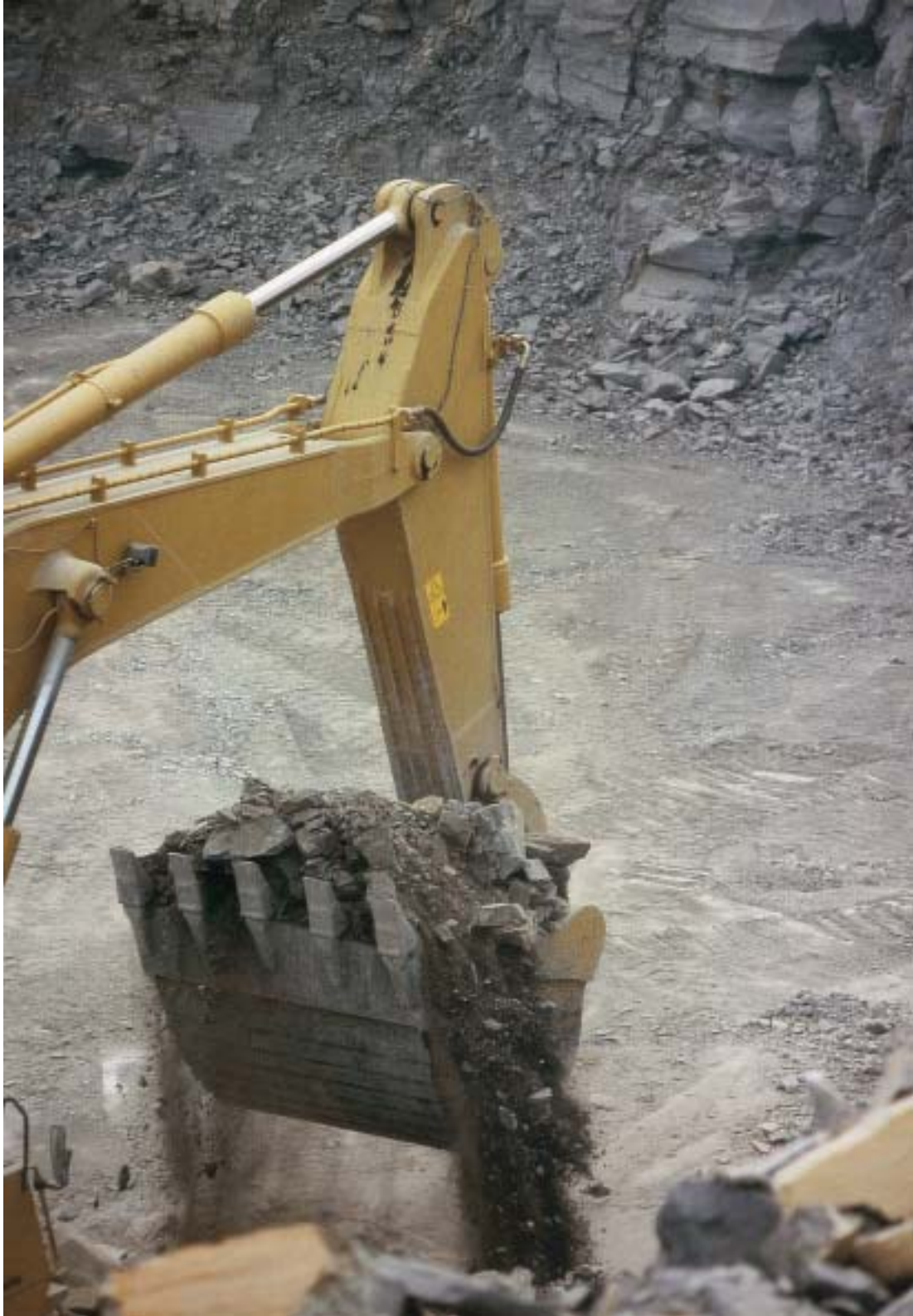
Figure 1: Excavator shovel made of DILLIDUR-V steels in the harsh conditions of open-cast mining (Illustration used with the kind permission of Schlüter Baumaschinen, Erwitte, Westphalia, Germany)
